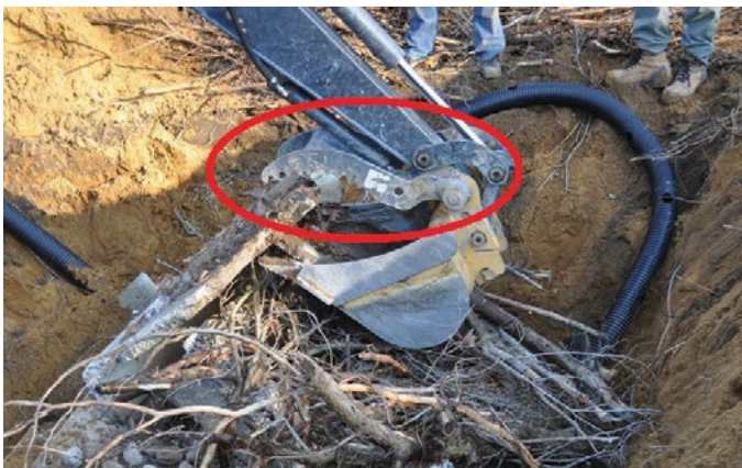
Figure 12. An excavator bucket with a “thumb” has more control in placing materials within the hibernaculum. © G. Beck
