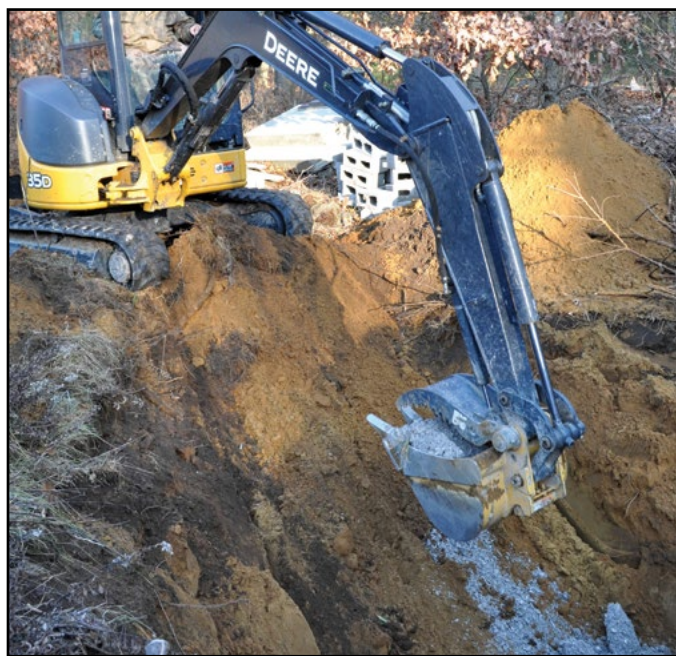
Figure 6. Dumping a sand/gravel mix into the bottom of the excavated hibernaculum to promote drainage. © G. Beck
