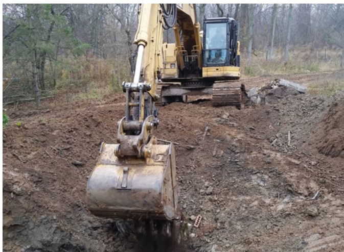
Figure 4. A large excavator digging in the early stages of hibernaculum construction. © G. Beck
