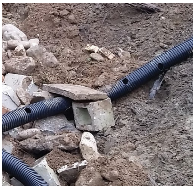
Figure 7. Early in the construction process, arrange "Big O" plastic pipe from the bottom of the excavation to the surface. Drill large diameter holes into the pipe to increase air circulation and to provide potential entry/exit spots for snakes.
