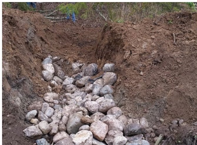
Figure 5. An overflow drainage spillway during mid-construction, built to mitigate potential rapid flooding of the constructed hibernaculum. The spillway is built above the grade level of the deepest part of the excavated "bowl" to allow some water to remain within the hibernaculum. Field stone surrounds a Big 'O' pipe and will be covered with additional fill. © G. Beck
